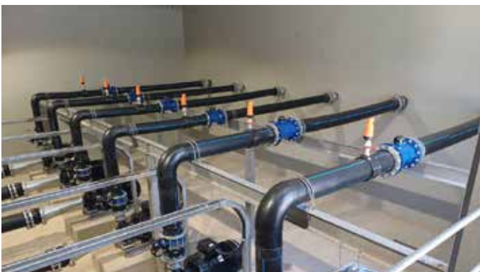
BOOSTER: AgriTurf designed, Tribinex built booster pump station.
