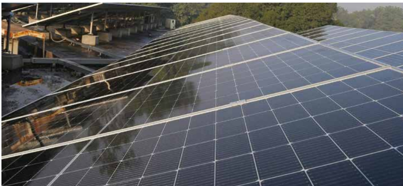
EMBEDDED GENERATION: The growing importance of embedded generation in Namibia's evolving electricity supply industry has necessitated the need for regulatory clarity and compliance.
