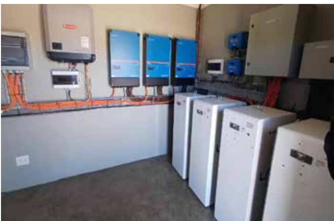
BACK-UP: Pump power room with backup solution for the control system.
