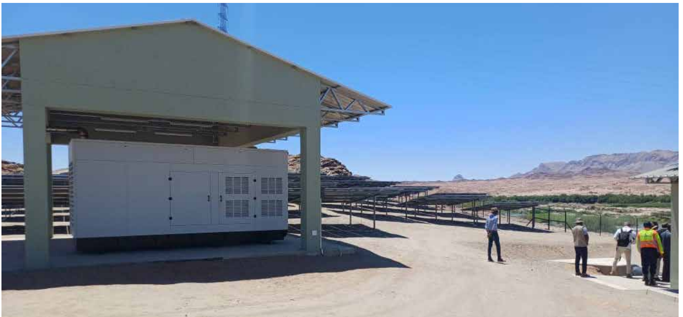
BACK-UP: 100% off-grid farm supported by a 500 kVA backup generator installed by NEC Energy, ensuring continuous pumping even on cloudy days or during high demand.
