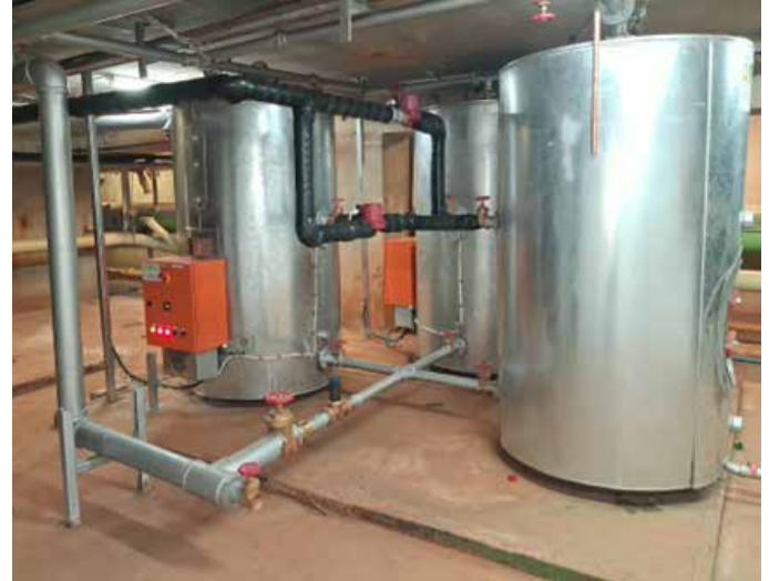
HOT WATER: Service floors fitted with three 12kW geysers
