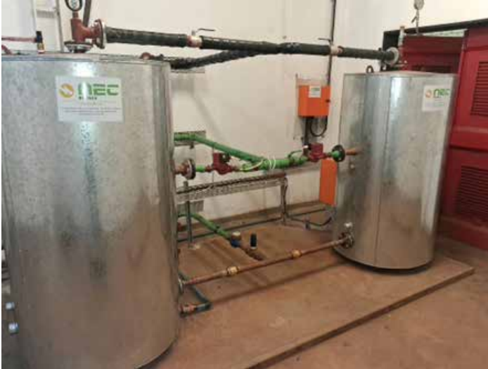
BOILERS: Two boilers providing hot water to kitchen
