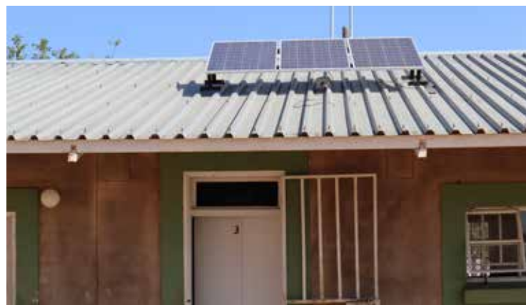
HUMBLE BEGININGS ... Mini-solar system donated by community members at Oomanya Combined School in Oshikoto Region.
