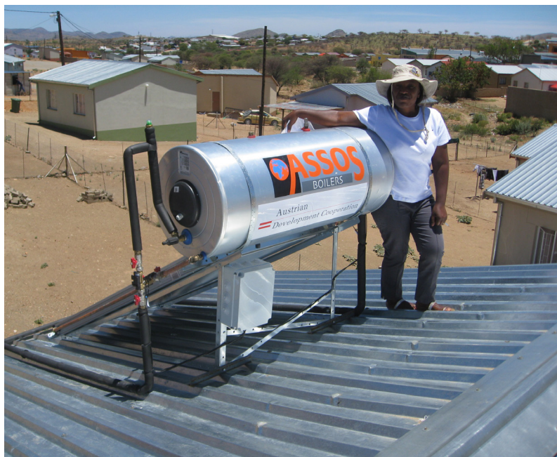
Helvi Iлека with a SWH installation at one of the NHE houses
