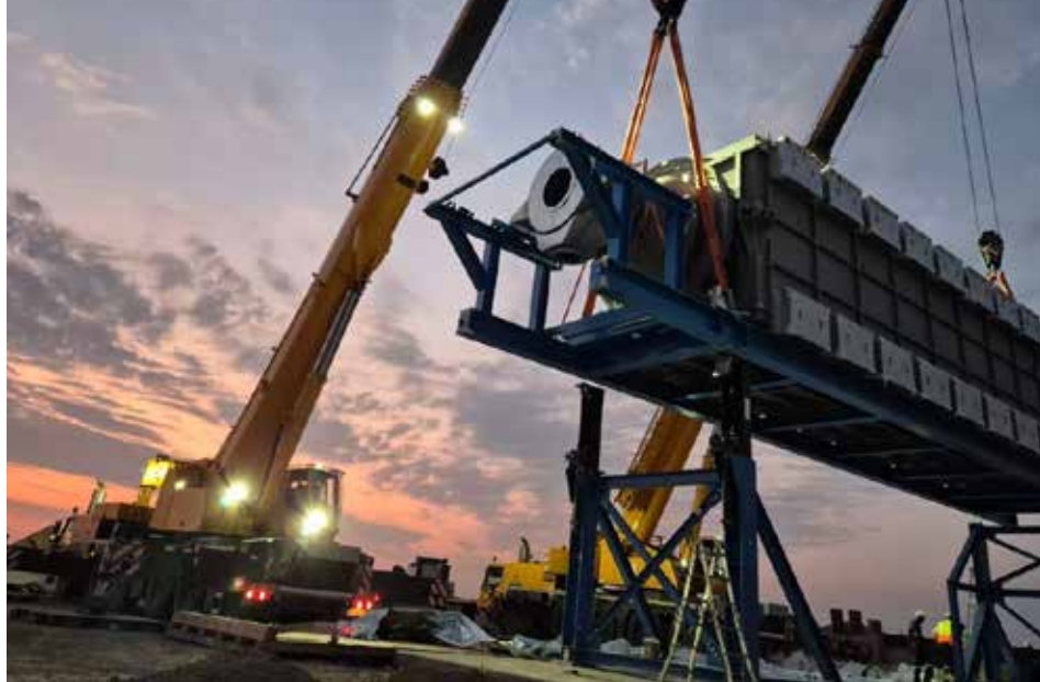
IN PRODUCTION: The HyIron production facility earmarked to start production by the end of February.
