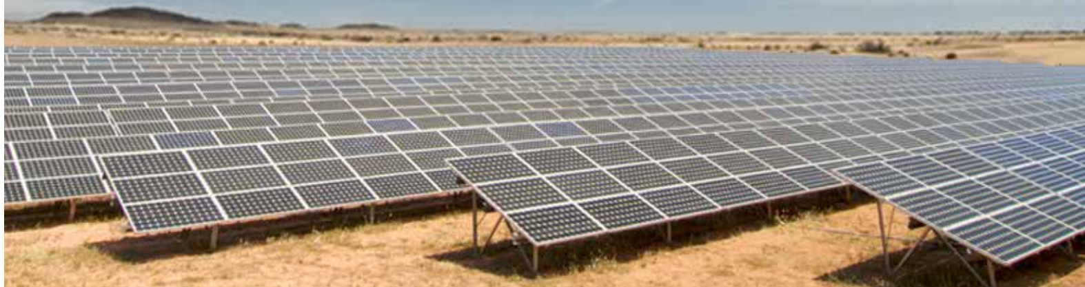
TeraSun Energy PV site
