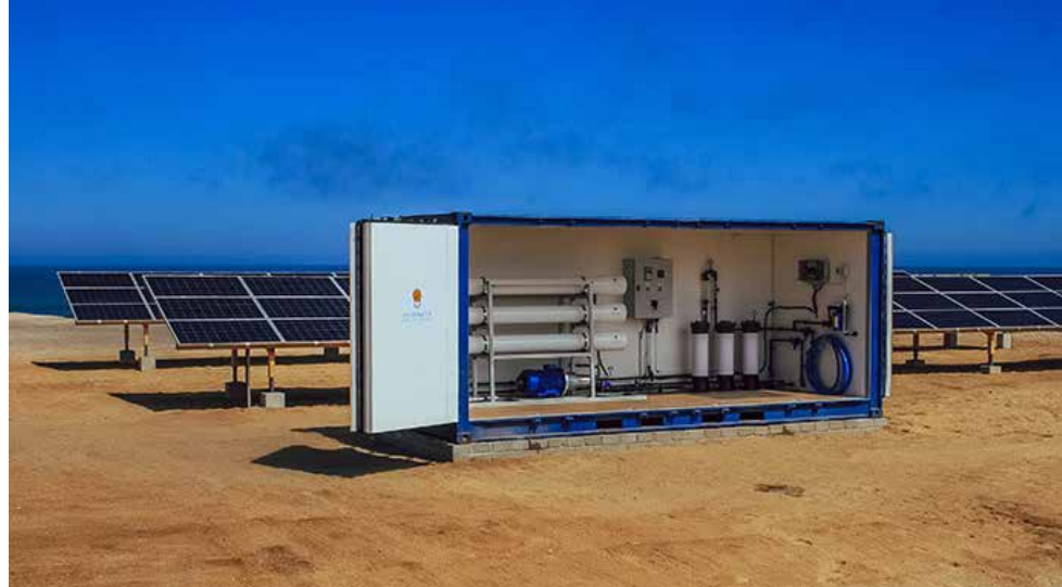
UNAM's desalination system has zero energy costs
