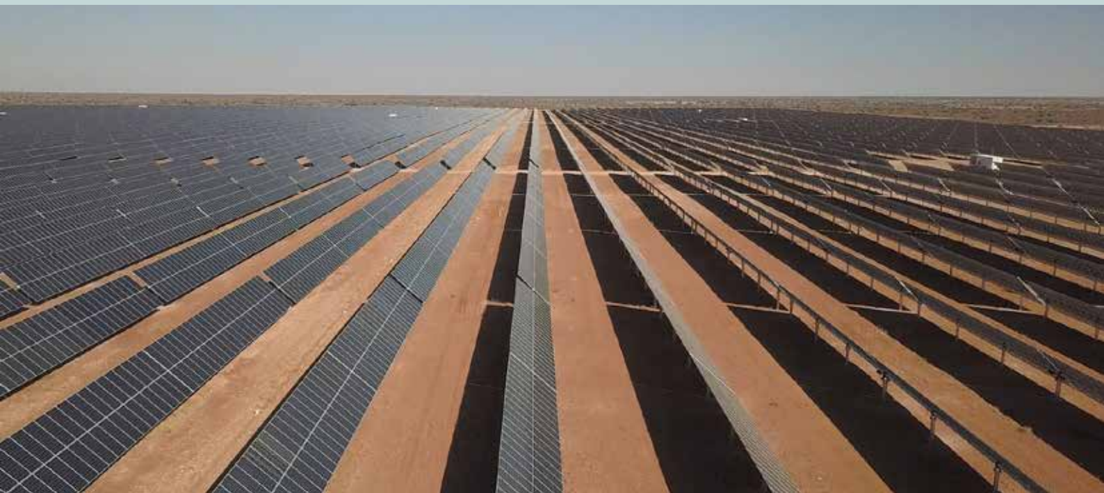
The gigantic Hardap solar plant outside Mariental. Photo by Conrad Roedern
