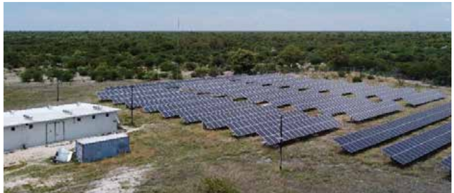
A 25.8 kWp solar PV decentralised system installed to complement the 300 kWp Tsumkwe Mini-grid. © TH Ingolstadt, Germany
