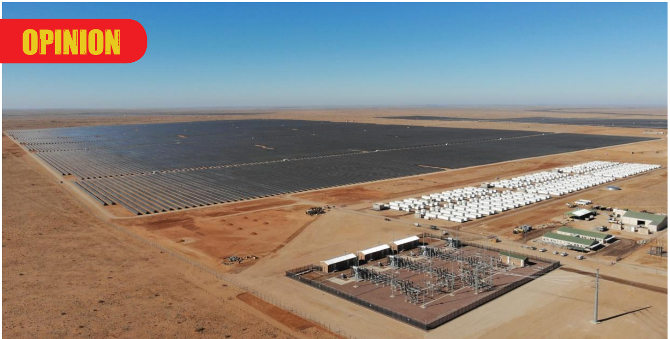
PACE SETTER ... The 530MW/1140MWh Scatec complex near Kenhardt in South Africa. Photo: Scatec
