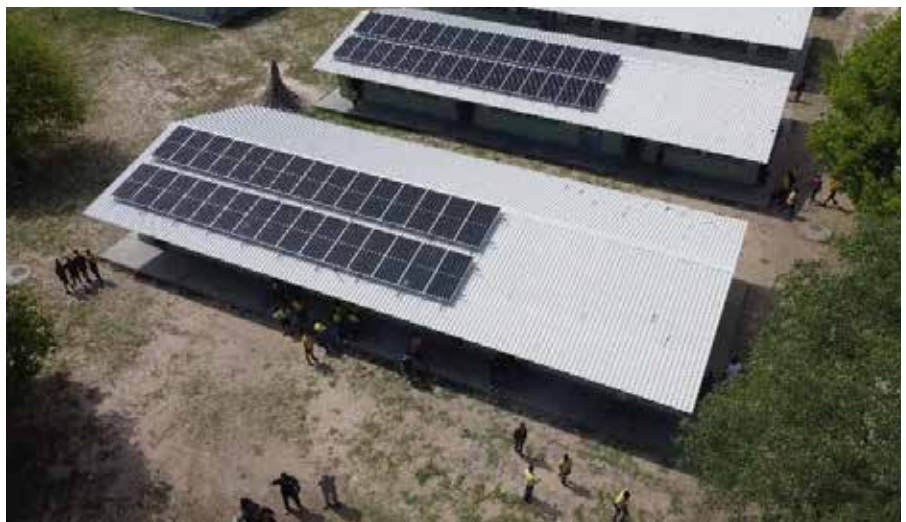
The decentralised system at Tsumkwe Secondary School. © TH Ingolstadt, Germany
