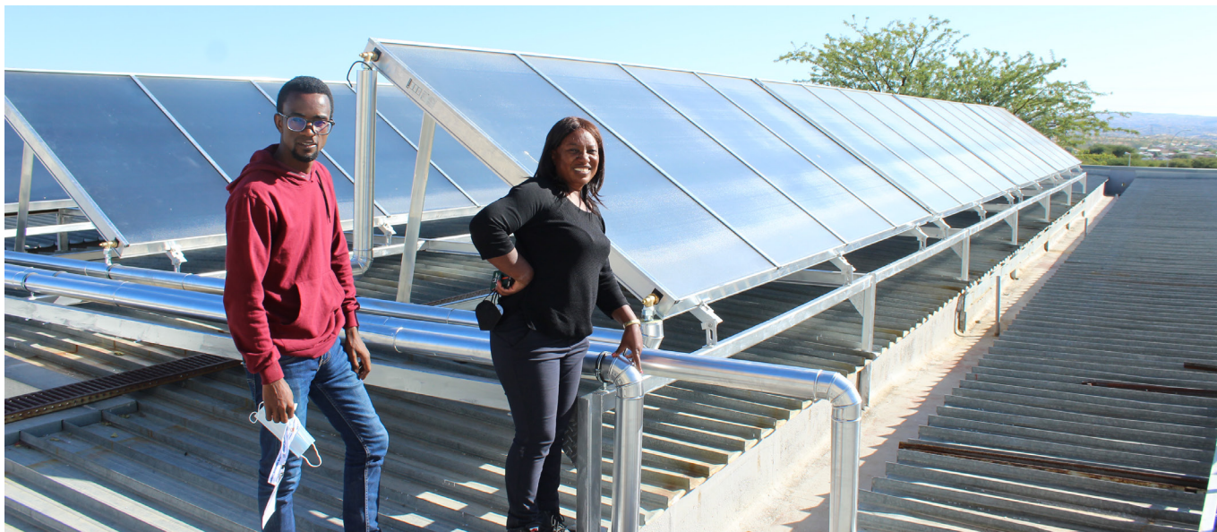
SUN POWER ... NEI Acting Head Helvi Ileka and NUST lecturer for Mining, Mechanical and Process Engineering Frans Hanghome in front of collectors of the 84kW solar water heating system installed at Katutura Hospital Maternity Ward.
