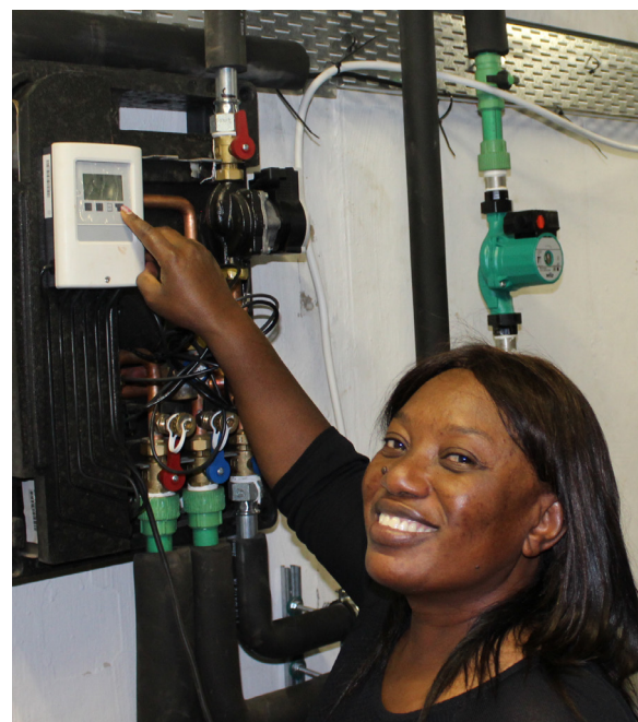
HOW IT WORKS ... Helvi Ileka explaining some of the modern components of the new system
