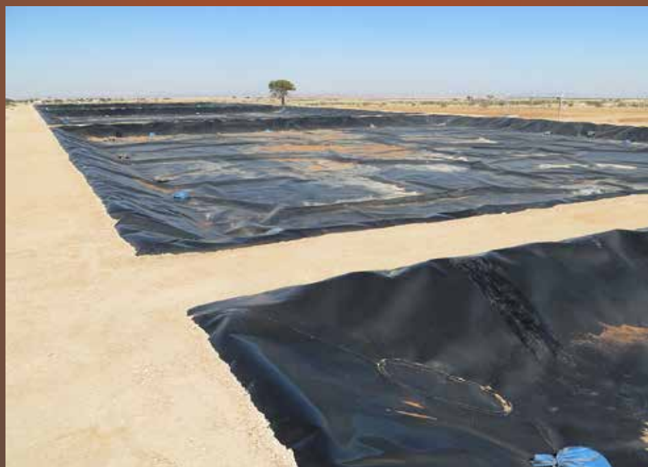
PILOT PROJECT ... The Groundwater Desalination Plant at Grünau, in the //Kharas Region. Photos: Kuchling Consulting Engineers
