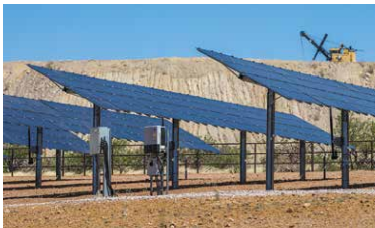
ENVIRO FRIENDLY: B2Gold aims to reduce its carbon footprint and its reliance on a heavy fuel oil (HFO) power plant with the new 7 megawatt solar photovoltaic plant at the Otjikoto Mine
