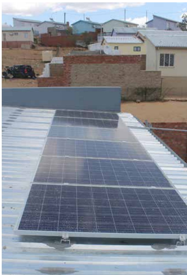
A 1.59kW photovoltaic module was installed to directly power a resistive element for heating the 300L tank using direct current without an inverter
