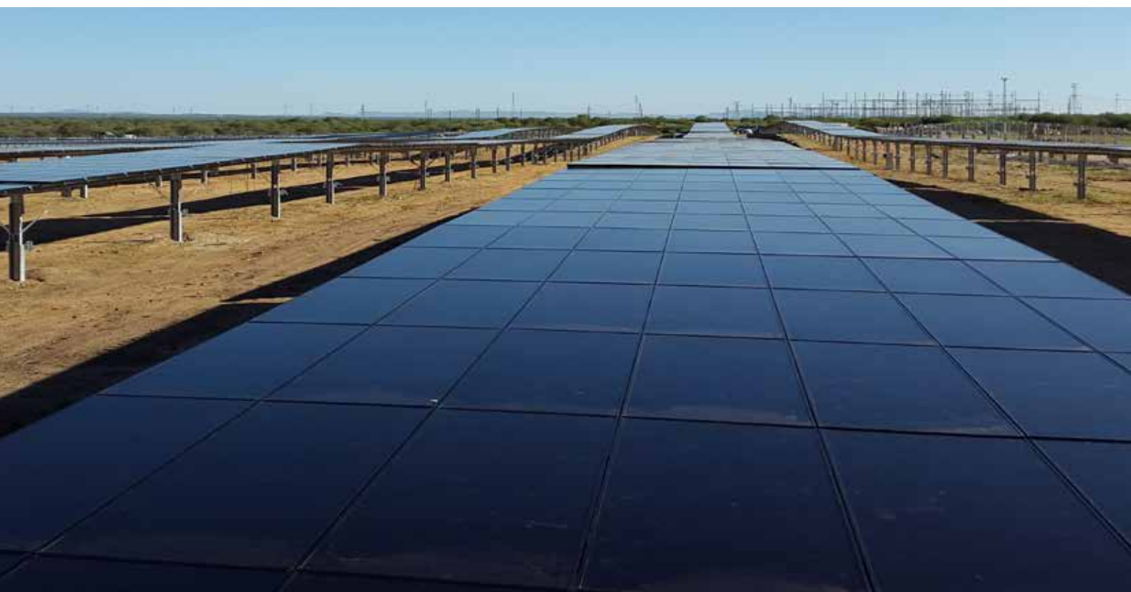
Omburu is currently home to this 4.5MW solar plant developed by InnoSun in 2015
