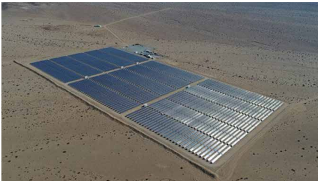
The 5MW Rosh Pinah solar PV plant
